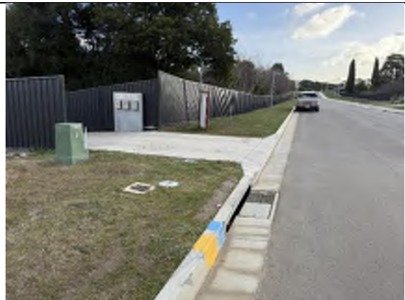
Figure 18 – Existing hydrant on Fermoy Lane. Within 120m of lots 2-5.
