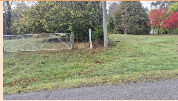
Existing fire plug to southeast
