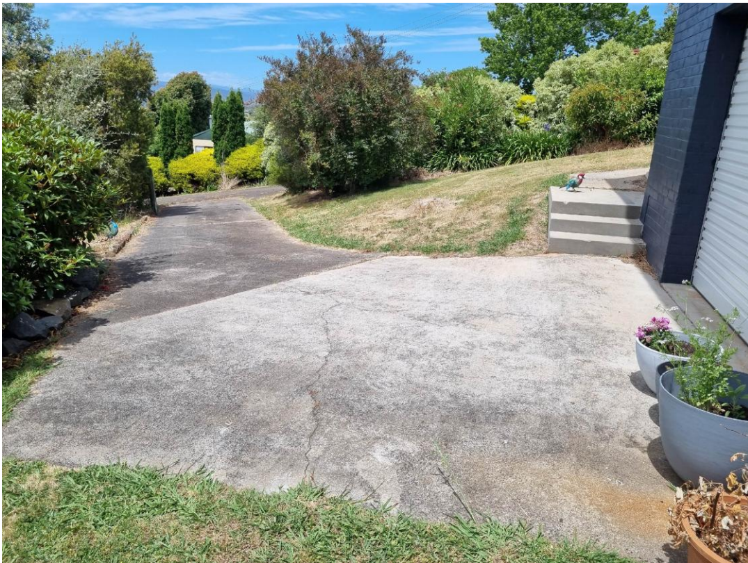
Photo 8. Cracking in existing concrete driveway, looking southeast.
