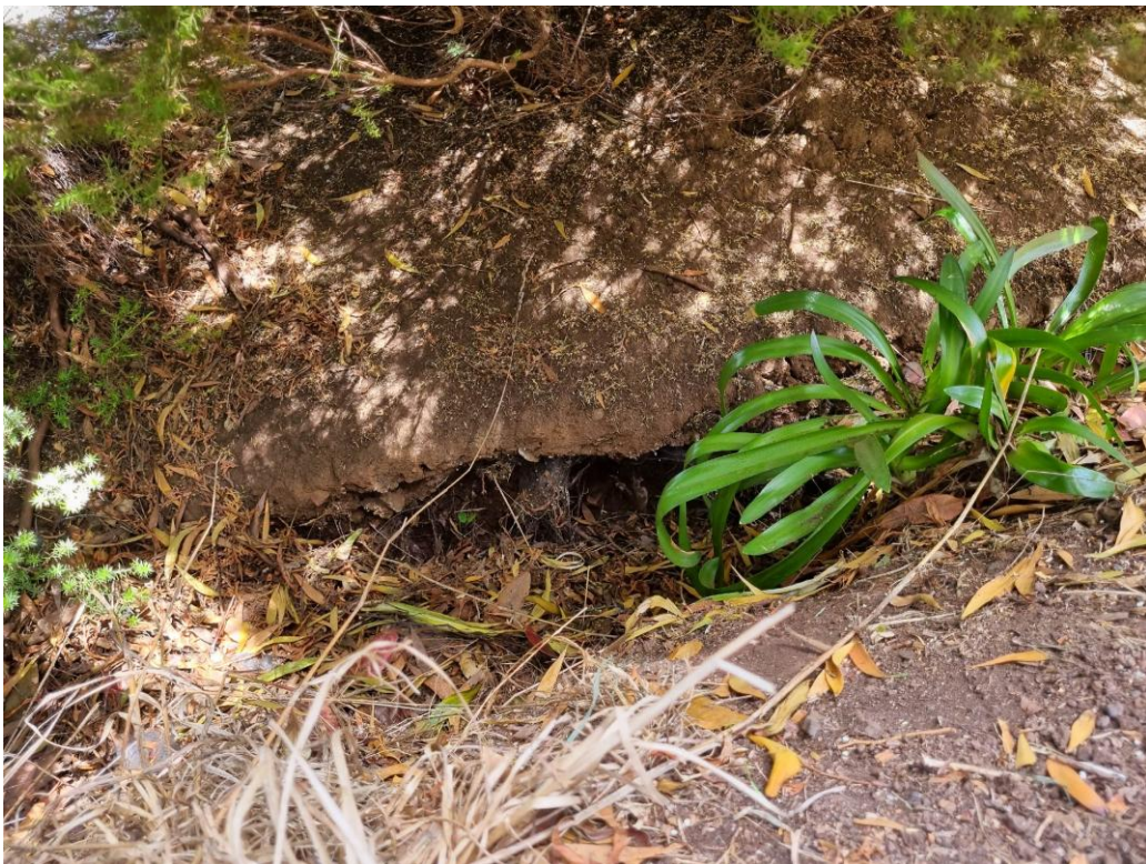
Photo 12. Erosion in unlined table drain on southern side of existing driveway.
