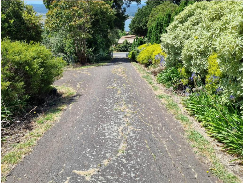
Photo 9. Cracking in existing asphalt driveway, looking northeast.
