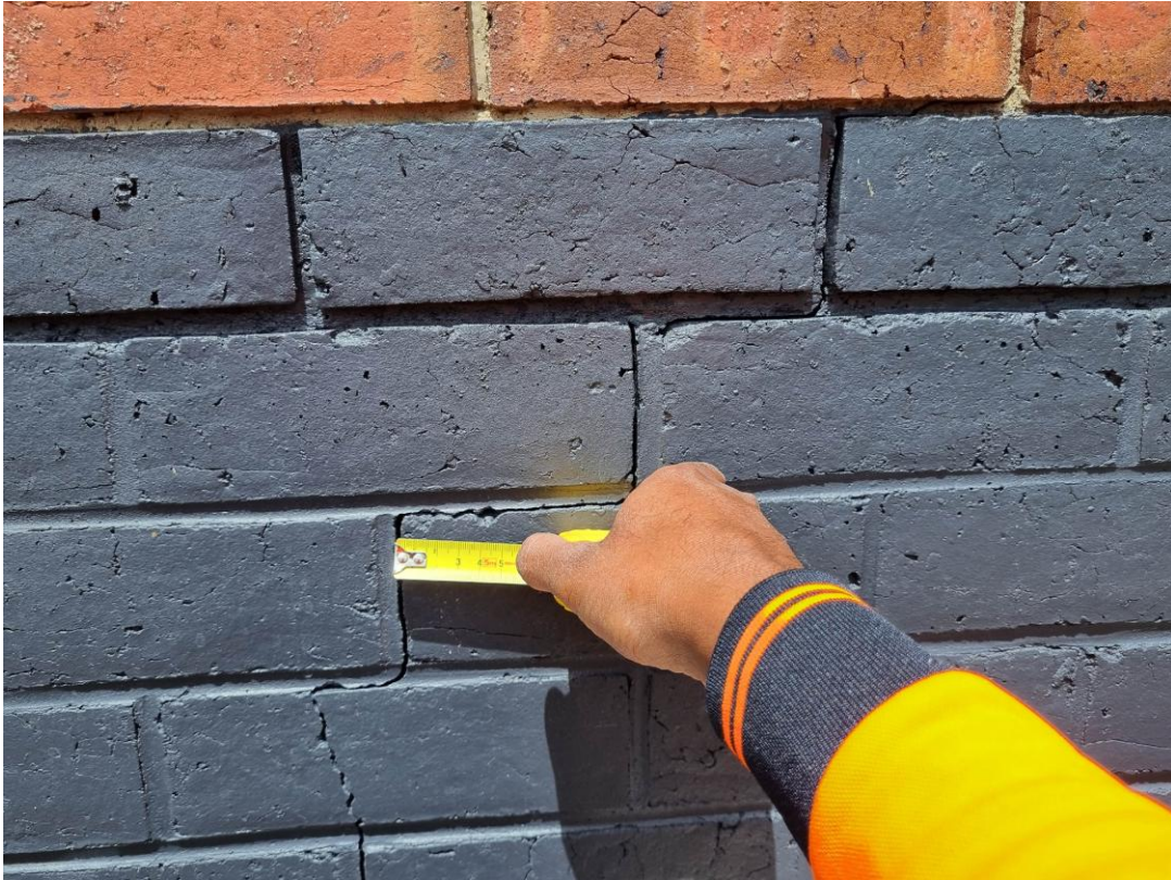
Photo 7. Cracked brickwork in north-western wall of existing dwelling.
